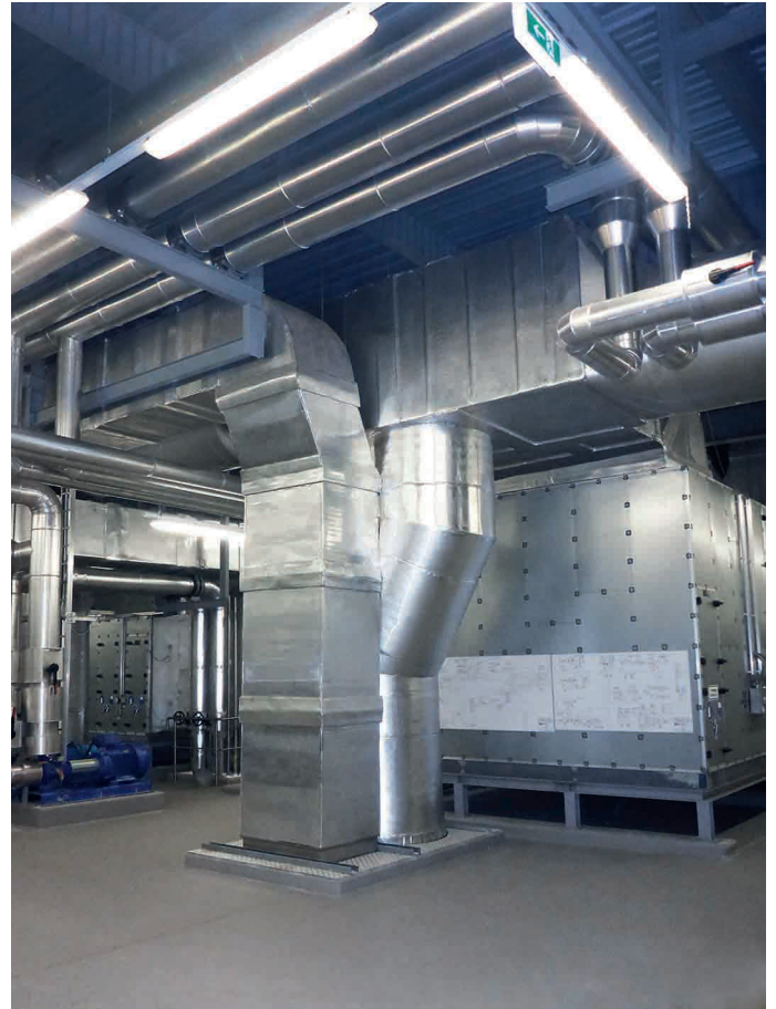
The central air-handling station is located on a separate floor under the roof of the new building
