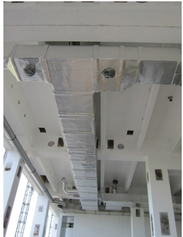
The air-ducts in the production hall are exposed to very high temperatures and 70 % humidity
