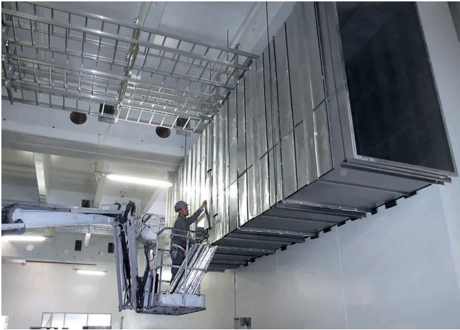
Some of the huge air ducts run at dizzying heights and can only be reached with a manlift
