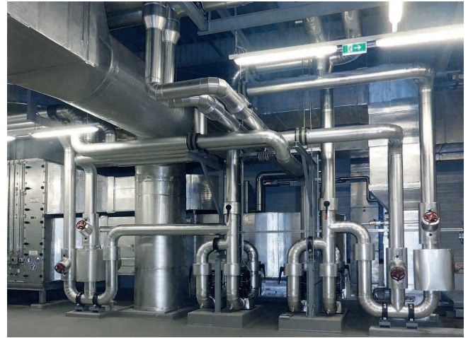
Armacell's pre-covered elastomeric insulation material, was specified for insulating all pipes and ducts of the air-handling system
