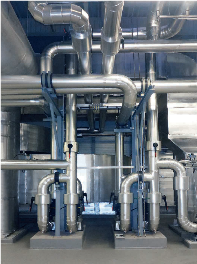
The ventilation installations were insulated with around 10,500 m 2 of Arma-Chek Silver sheet material
