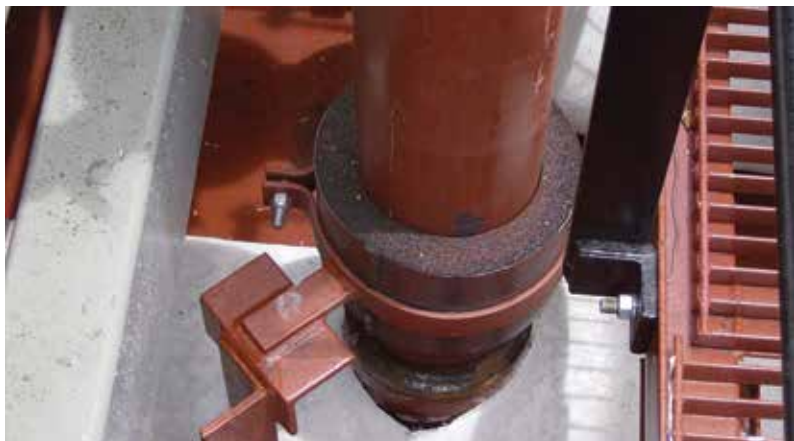
NH/Armaflex has been used on the majority of the technical insulation on the T-AKE ships.
