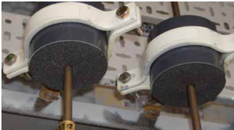
On the T-AKE ship USNS William McLean PCI used several hundred Armafix NH pipe supports on various cold lines.
