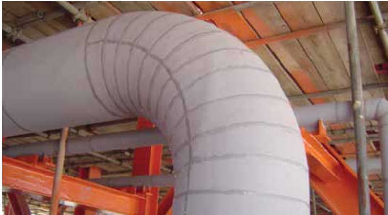
Finished bend at Ammonia-Urea-Melamine (AUM) complex.
