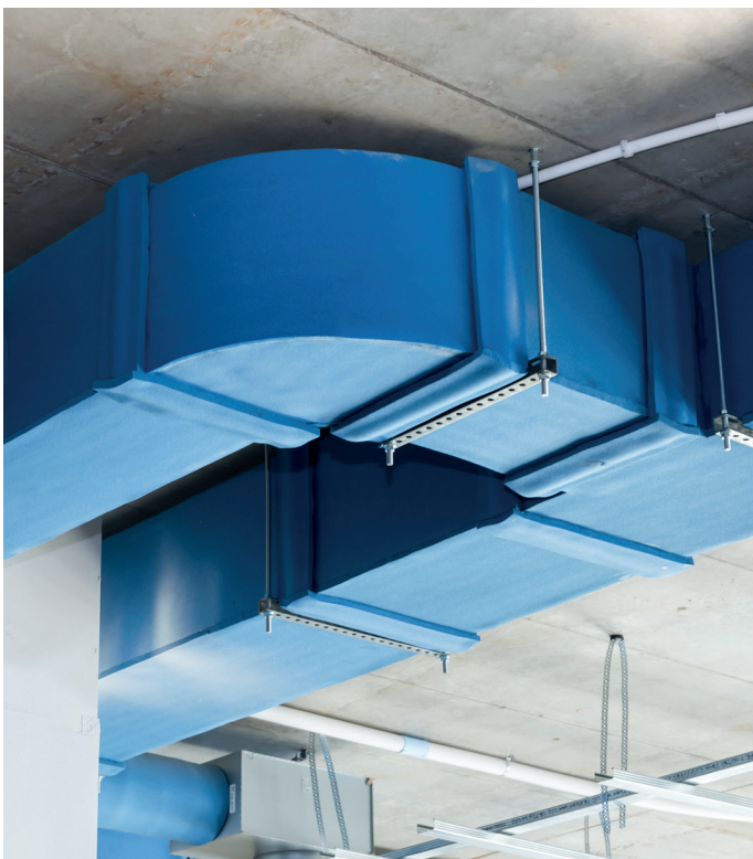
The air ducts were also insulated with the new elastomeric insulation material, which develops significantly less smoke in a fire than traditional FEFs
