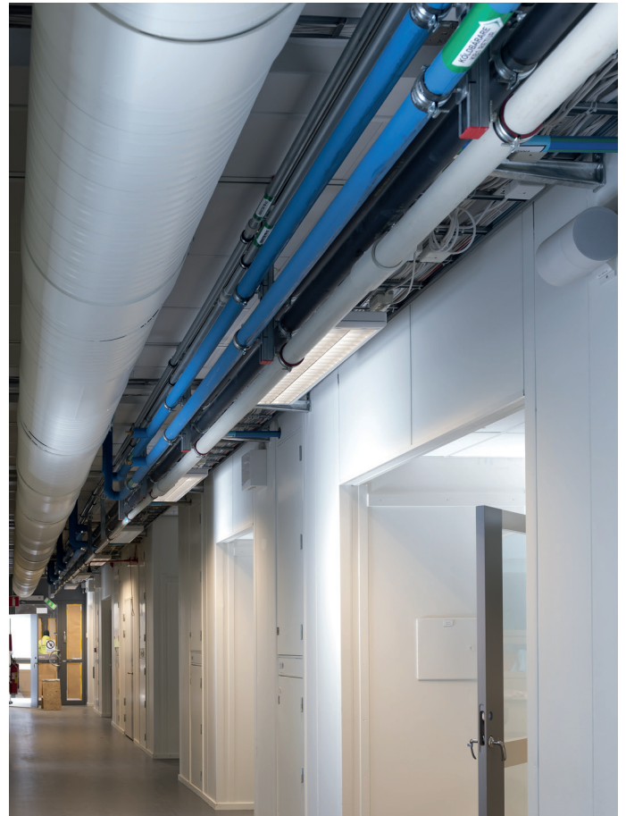
Armaflex Ultima is listed as non-hazardous by Byggarubedömningen (BVB), the Swedish institute that assesses the sustainability of building materials - an important selection criterion for this demanding project
