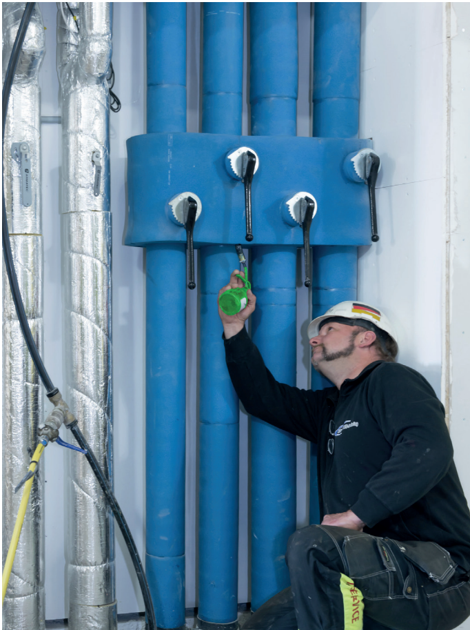
The employees of Knivsta Isolering AB installed around 2 500 m of Armaflex Ultima tubes and 1 000 m 2 of sheet material in the Skandion Clinic
