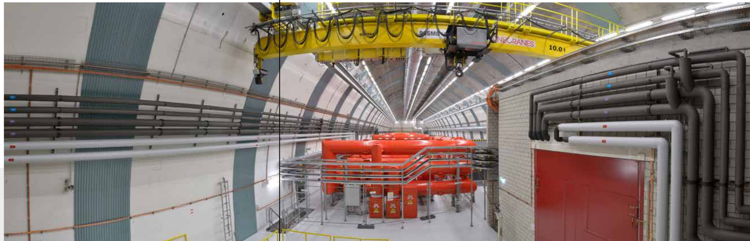
The machine transformers à 280 MVA each are housed in the slightly smaller transformer cavern.
