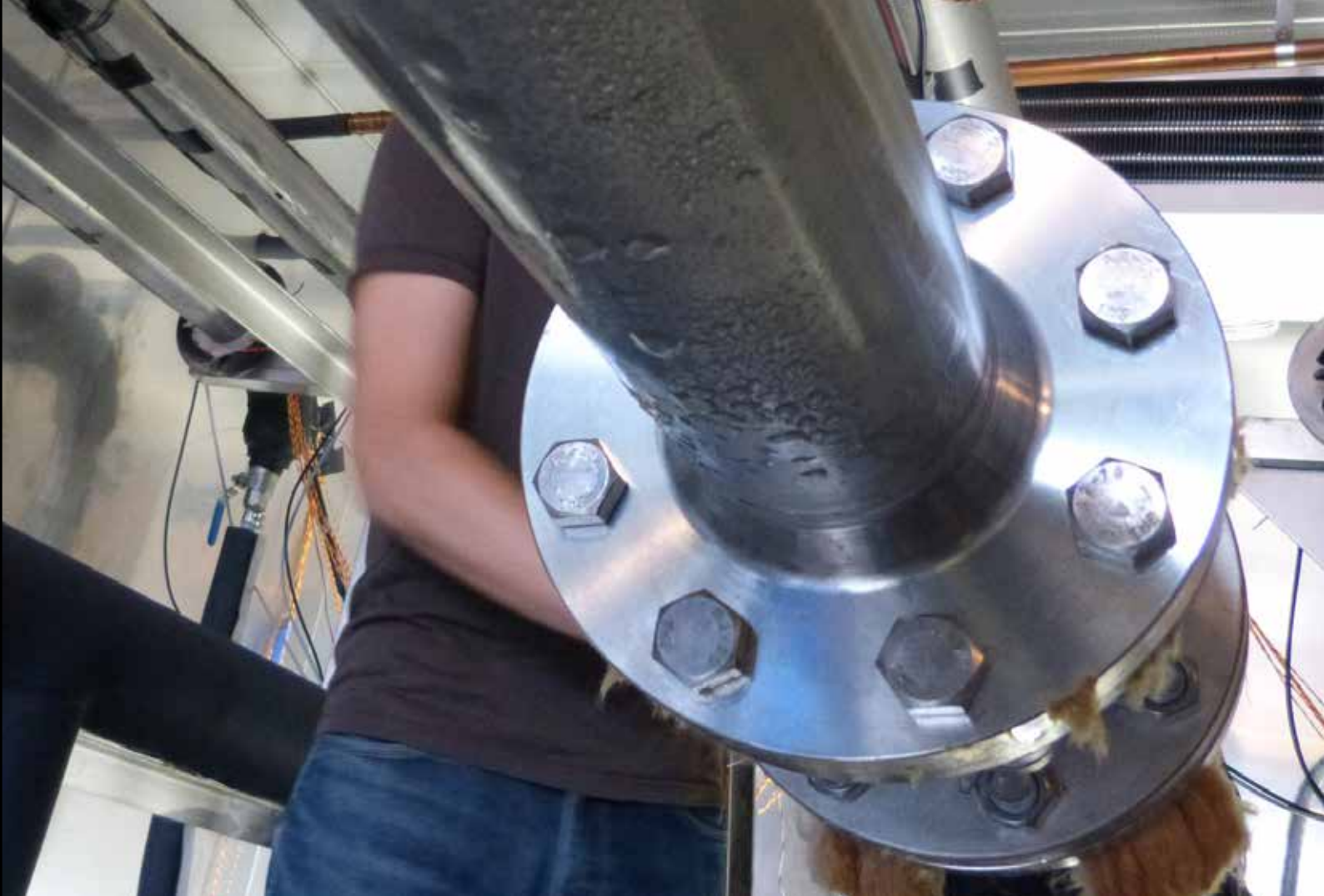
Figure 6: In the case of the mineral fibre insulation, humid air has penetrated especially around fittings, yet even these areas have remained dry under the FEF insulation.
